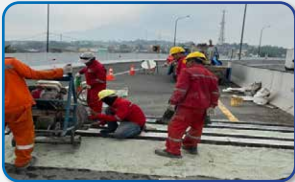
Pekerjaan Rekonstruksi Rigid, Laston, Overlay dan Expansion Joint Reconstruction of Rigid, Laston, Overlay and Expansion Joint
